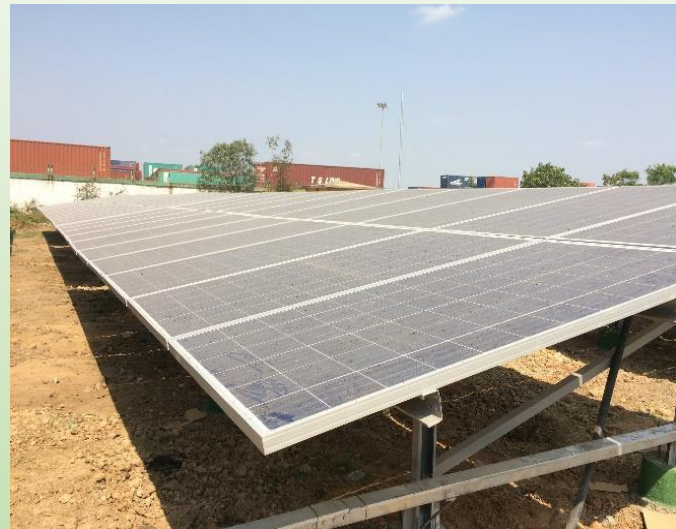
200 KWp solar plant at Manali, Chennai
